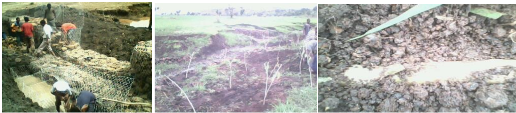
Fig. 4. Gabion check dam construction and planted branch cuttings by direct and layering on reshaped gully
